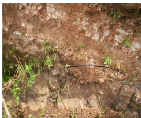
Figure 7. Photo of weathering appearance which is controlled by a system of cracks, (Source: Suwarno, 2014)
