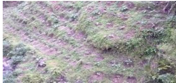
Fig.8. Photos of surface erosion appearance, (Source: Suwarno, 2014)
