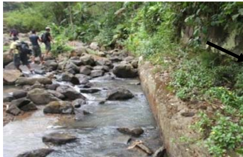
Fig.4. The appearance of a fault (Source: Suwarno, 2014).
