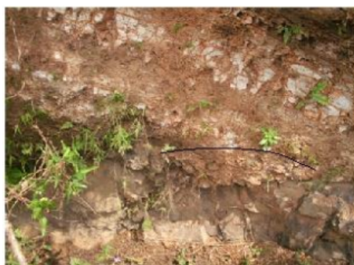
Fig.7. Photo of weathering appearance which is controlled by a system of cracks, (Source: Suwamo, 2014)
